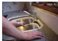
Trial fit sink to ensure tap flange is clear of sink rim.
