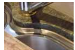
Tap pad shows oversize cut out. Sink wont align with granite edge.
